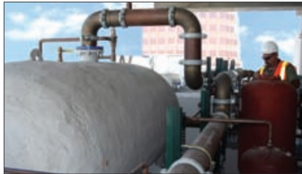
Bill Siler inspects a hot water heater installation at a high rise condominium.
